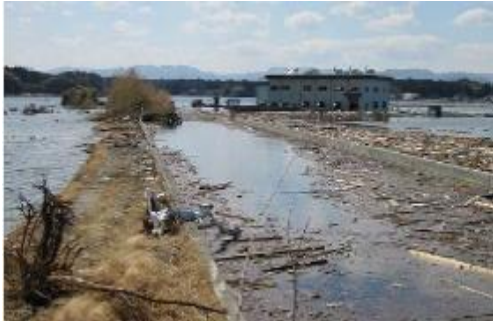
Tsunami-damaged drainage pump station and submerged farmland
